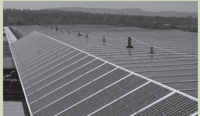
Solar panels at Portland International Airport
